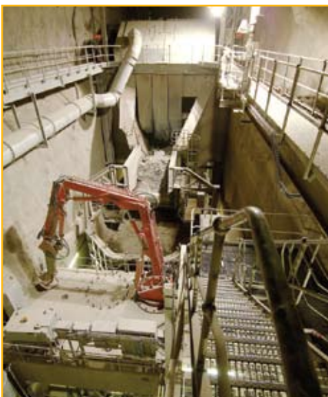
Underground crusher with rock breaker.
